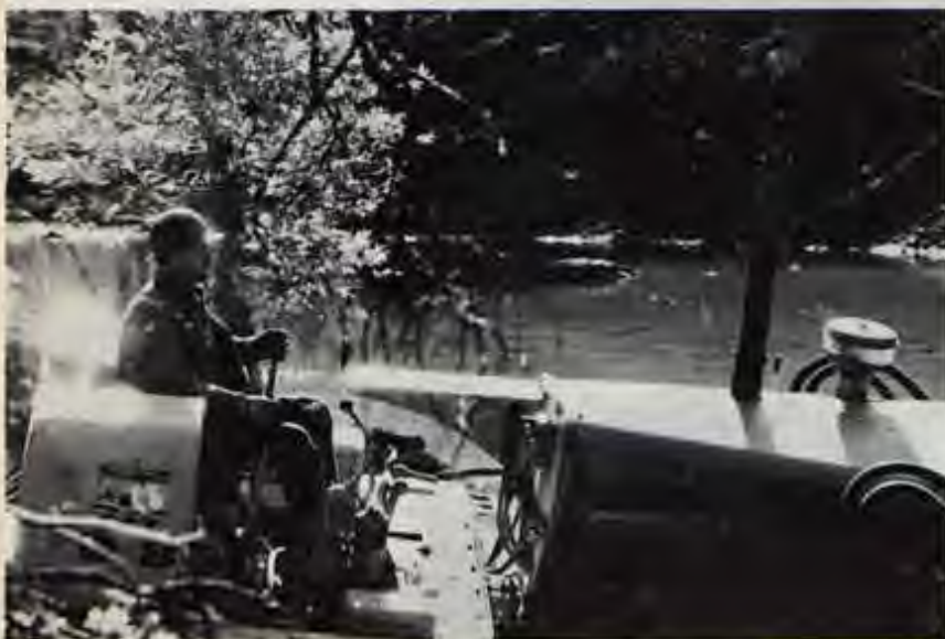
Bulldozer operator Eldin Pura widened Tassajara Creek to divert and slow down its flow.
